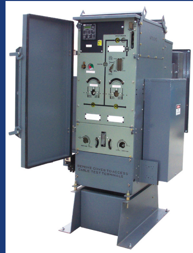
22000V 400A ring main unit with 200A circuit breaker fitted with Orion IPR-A over current and earth fault relay
