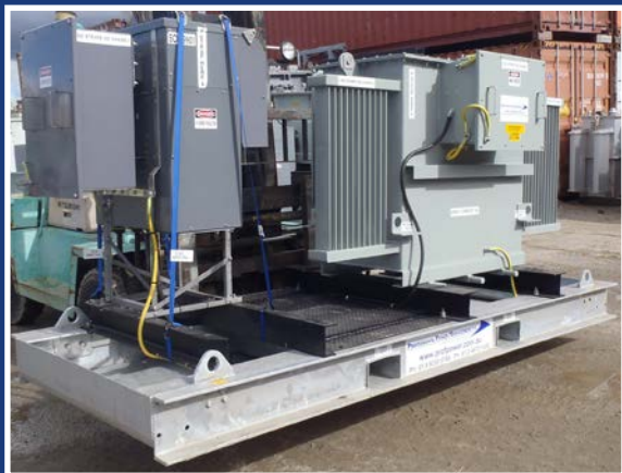
500kVA 440 / 11000V step up portable substation fitted with OC/EF/EL protection. Assembled onto oil containment base.
