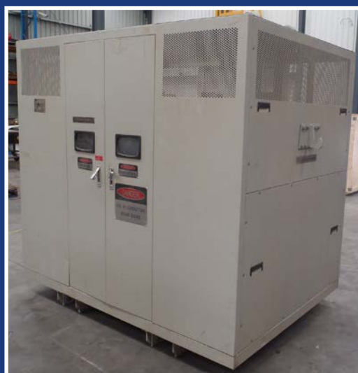
1500kVA 11000 / 433V Dry type transformer
